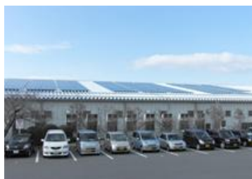
Solar panels installed at Shiga factory
